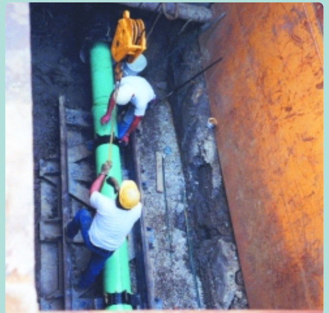
Two workers down in the trench joining the pipe sections and pushing the carrier pipe into the casing.
