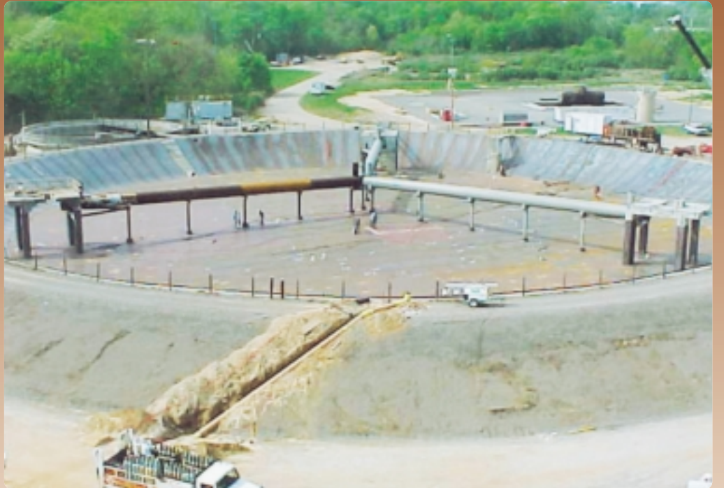
Installation at the caprolactam production plant of DSM Chemicals North America, Inc., near Augusta, Georgia.
