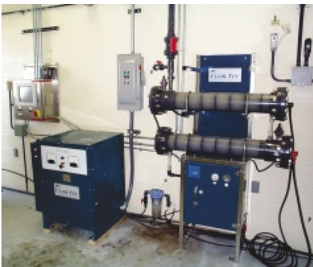
View of the Chlorine Room at AWUD's Gonzales station where a two-cell system was installed. A wall-mounted control panel is at the left, with the power supply/rectifier in the center and the electrolytic unit is at the right. ▲
