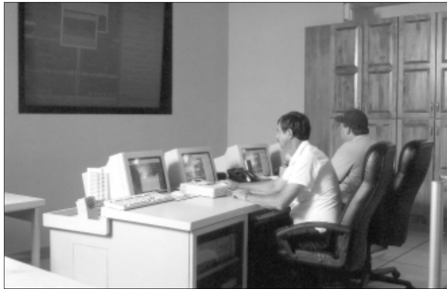
The Community Water System computer network provides a variety of important functions including the monitoring of all pumping station entrances and tank locks. If any unauthorized entry is attempted, the system immediately detects the activity and sets off an alarm.
