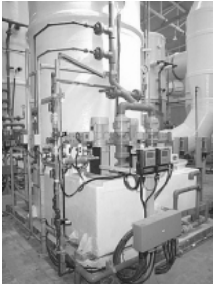
Figure 3: Odor Control Systems at the Odor Treatment Building
