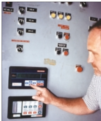
This recently installed liquid level control panel is a conductivity probe-based system that is fully compatible with the lift station's new SCADA system. Plans are to network eight stations with the SCADA to achieve a continuously monitored system.
