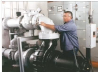
This 60-hp pump handles peak flows along with another identical pump. During low-flow periods, a third 20-hp pump takes over to reduce the station's energy consumption.
