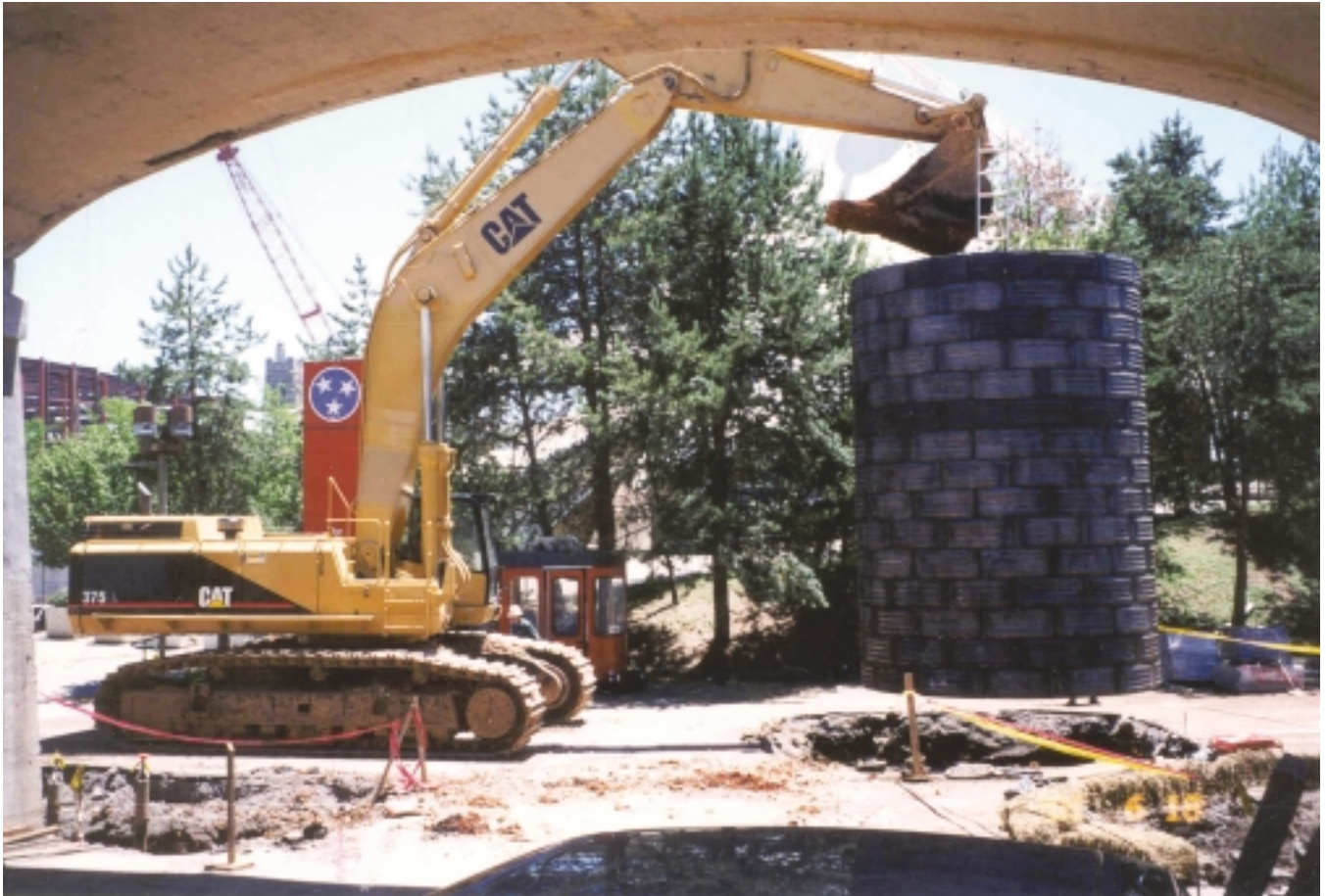
An open-cut method was utilized to install the 48" sewer pipe during Phase II of the project.
