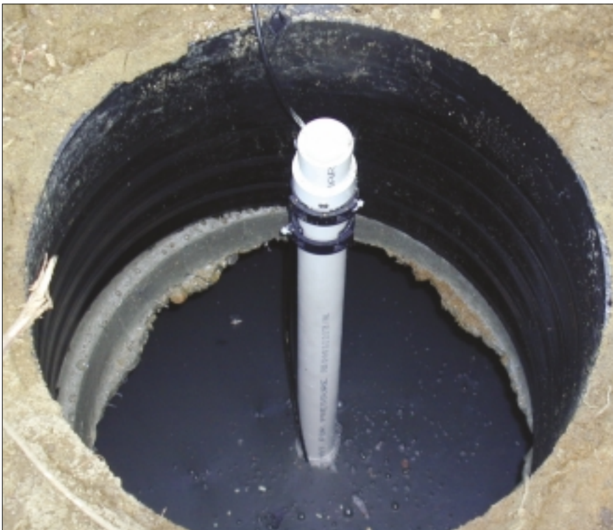
Manual measuring of sludge, grease and liquid levels is too costly and time consuming to do on a regular basis.
