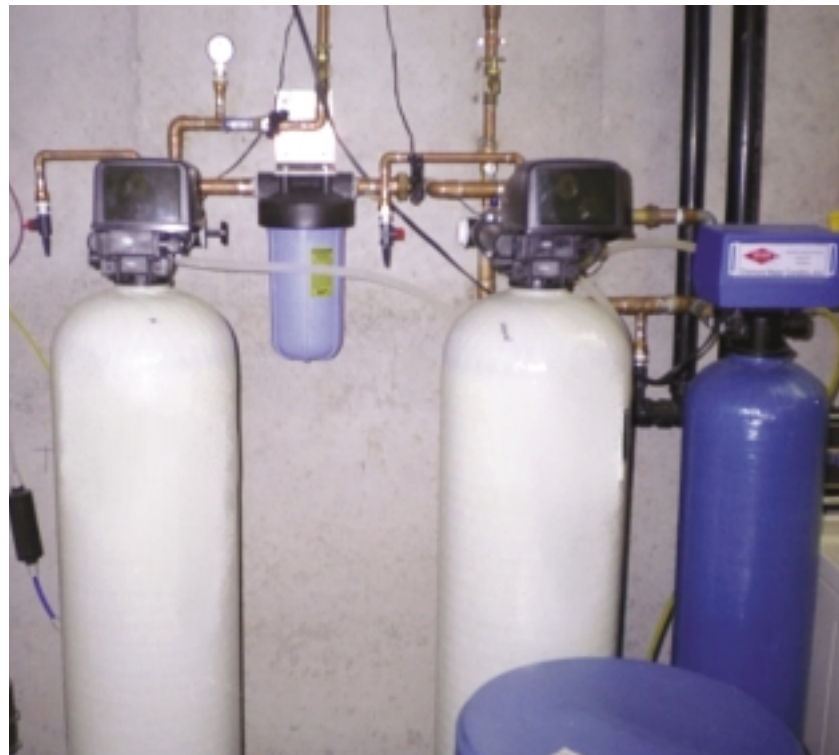
Typical POE arsenic removal system using Aqua-Bind adsorptive media.
