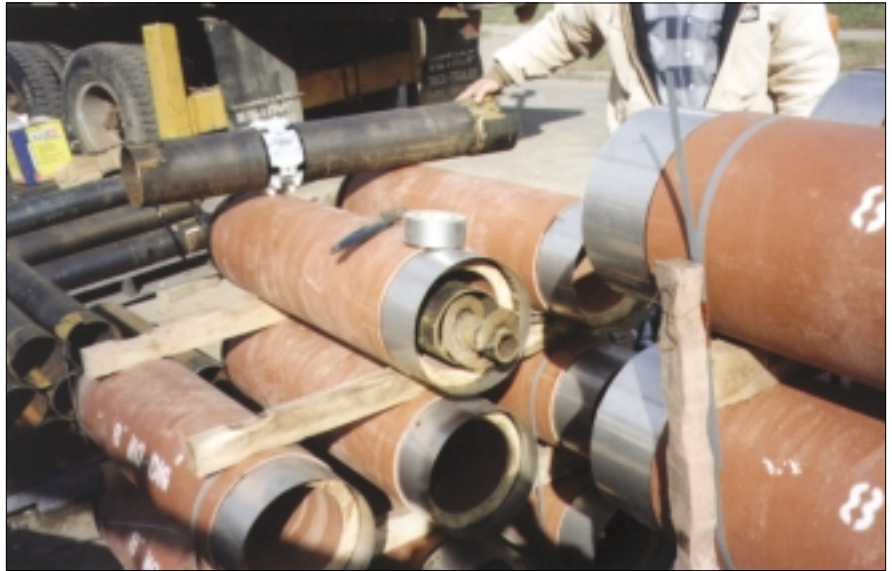
Sections of pipe await placement at one trenchless project. Increasingly, municipalities throughout the United States are specifying that contractors employ trenchless technologies for installing sewer and water lines.
