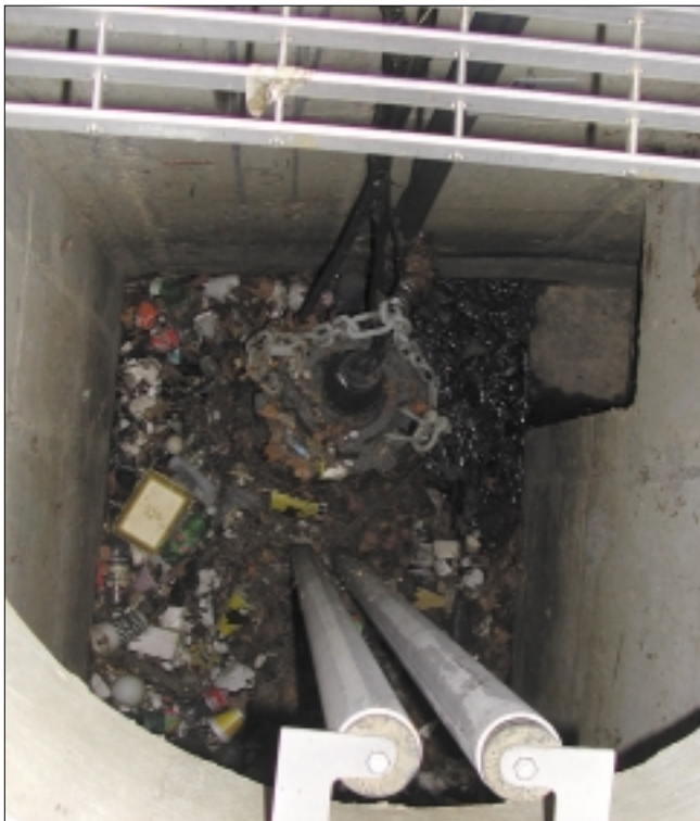
Up to four inches of sludge and trash may be left after the detention tank is drained. Chopper pumps must chew through this debris before it can be disposed.
