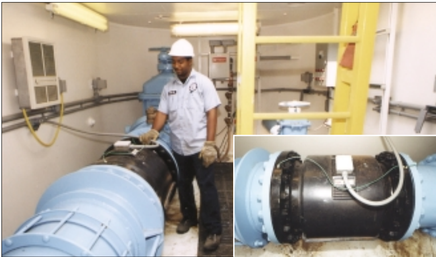
Figure 4: This underground vault houses the water meter sensor (inset). In the background, wall-mounted, is instrumentation that measures inlet and outlet water pressure and vault temperature.
