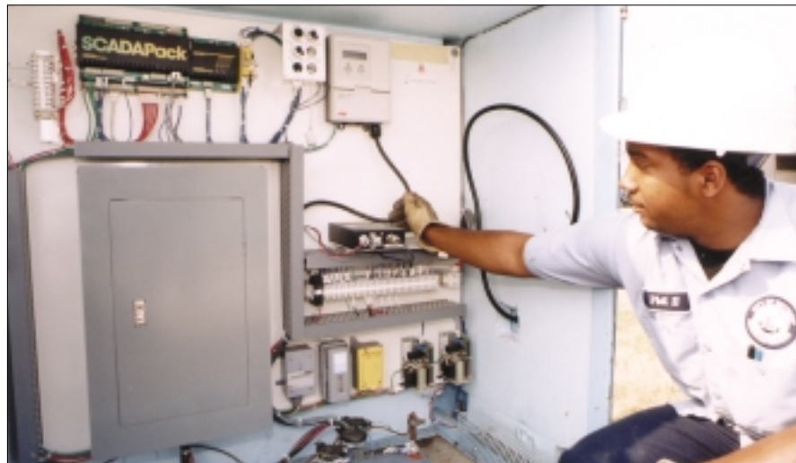
Figure 3: Philip Ellison, construction instrument technician, holds the cable that connects a transmitter to the sensor in the vault.
