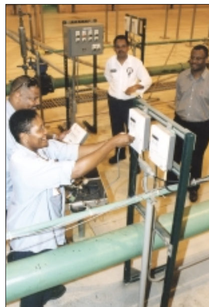
A CalMaster system is being set up in the test facility to check the calibration of one of the nine MagMasters. Shown clockwise are Marian Bryant, instrument apprentice; Greg King, instrument technician; Mashuk Meah, instrument technician foreman; and Rodney Johnson.
