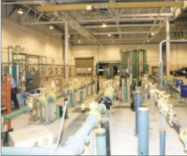
Figure 5: At the Detroit meter test facility, lines for test runs on different makes of meters vary in size from 1" to 12".
