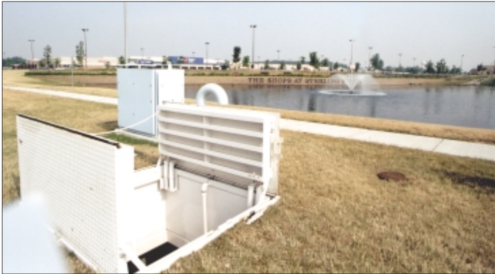
This is an above-ground view of the meter vault. The SCADA console is in back of the vault.
