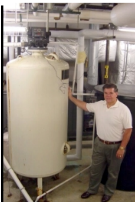
Kevin Britton (pictured), Quality Water of Maryland, worked with Duane Rinde, Director of Plant Operations at Glade Valley, to identify the problem and find a cost-effective solution.
