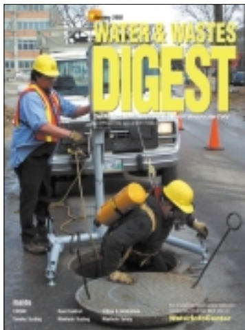
Cover: This manhole inspection crew is going down in search of damages caused by high sulfide levels. (Photo courtesy of the City of Winnipeg, Manitoba, Canada)
