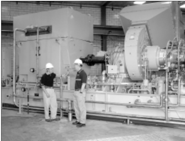
Two turbines generate electricity by burning the methane gas produced as a byproduct of the wastewater treatment process. Eventually, the plant may generate excess electricity that may be sold on the open market.
