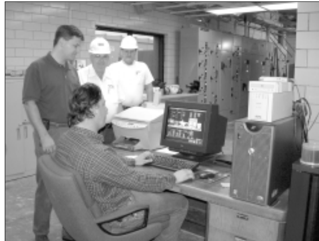
On-site technicians monitor the plant's energy-generating operations. Two gas-powered turbines also can be monitored remotely by personnel in a computerized control center in downtown Dallas.
