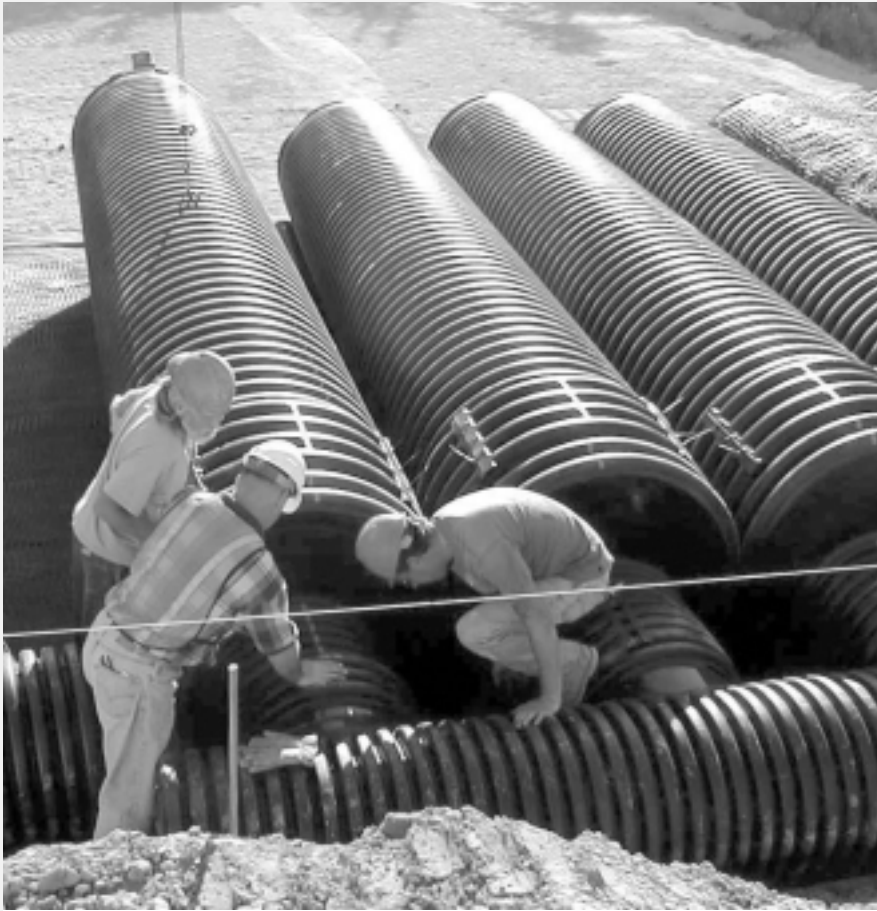
Along with eliminating the need to backfill and compact between 42" diameter lateral runs, the six-meter lengths and integral bell and spigot of N-12 pipe allowed installation of more than 450 feet per hour.
