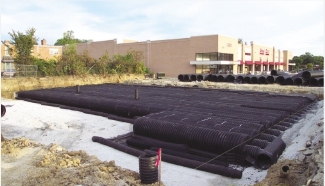
Installed in half the time of a traditional retention/detention system, the HDPE design meant minimal inconvenience to store patrons' parking needs.
