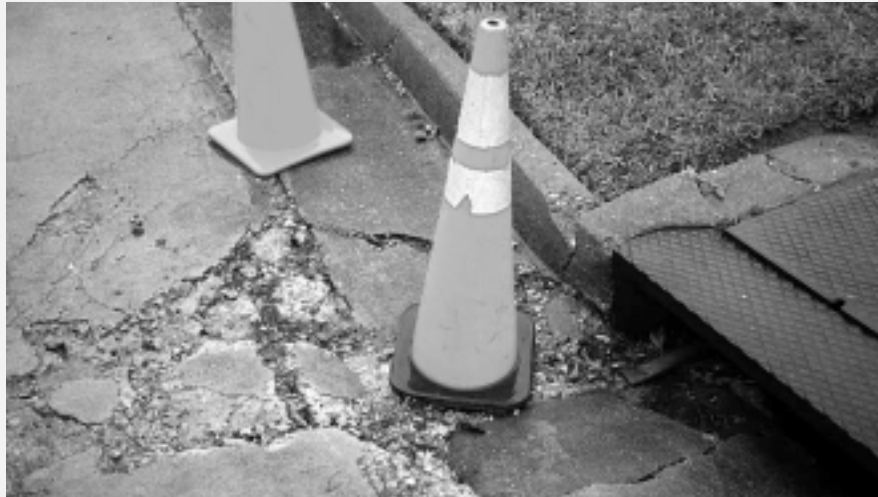
When notified of a cave-in, the City of Chesapeake responds quickly to eliminate any potential hazard.
