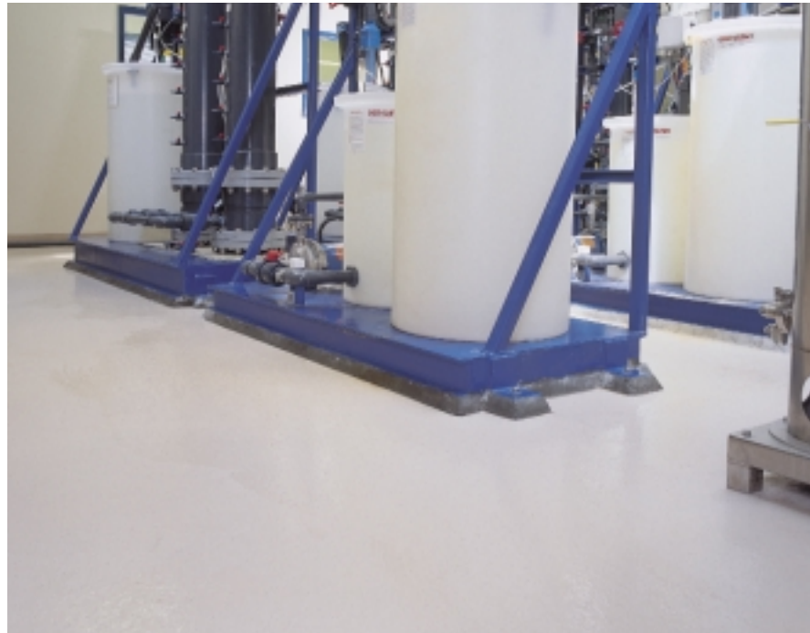
Floor coatings and overlayers protect the concrete flooring seen here in the pilot plant, located in the operations building. The pilot plant is a miniature of the entire plant operation; every process can be tested here for performance.
