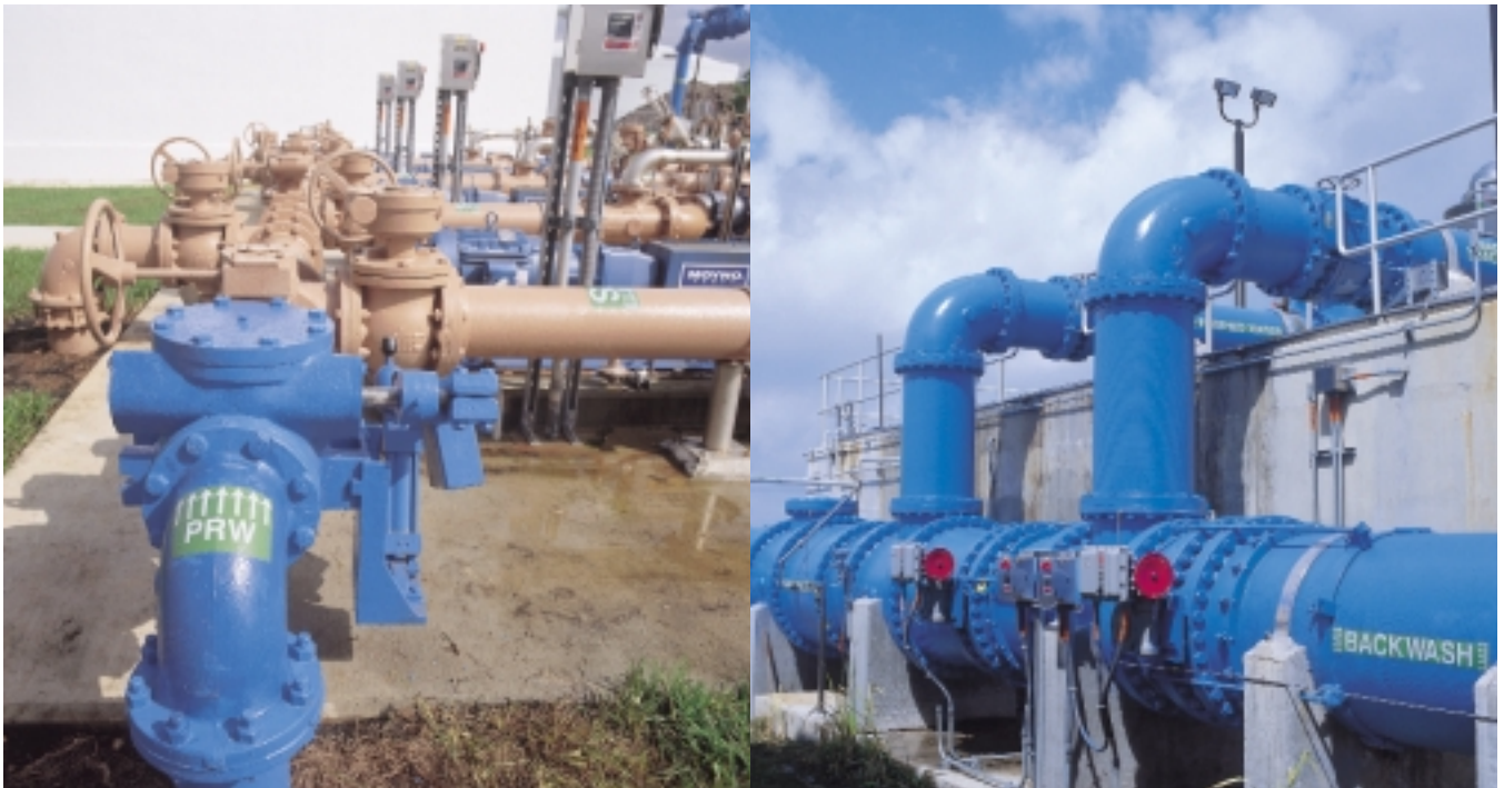
Color-coordinated, exterior steel coatings were used to protect and label the exposed piping seen here in the pipe gallery.
