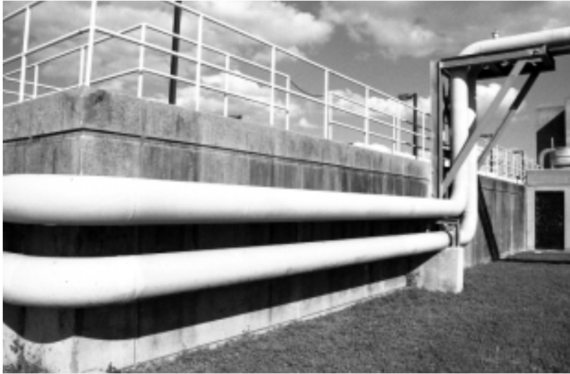
Cross-training into new job skills allowed Tampa's planned maintenance to double when compared to reactive maintenance.
