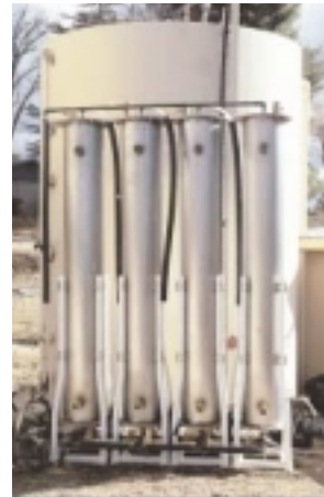
This arsenic removal system successfully reduced the arsenic level to below the new MCL of 10 ppb during the entire test period.
