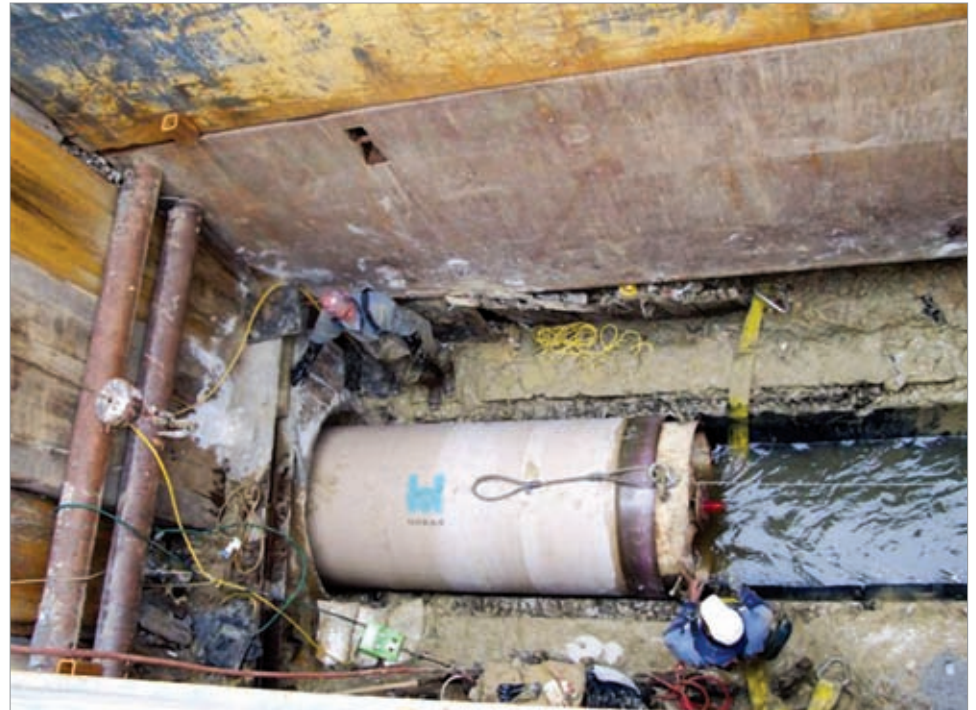
Allen & LeBlanc crew members slipline the 48-in. HOBAS CCFRPM pipe into position. The integral fiberglass low profile bell is gasketed and provides a watertight seal with the spigot joint while allowing the pipe to be pulled or jacked into the host pipe. The low profile design prevents hang-ups and minimizes friction during installation. The entire project was approximately 400 ft long.
