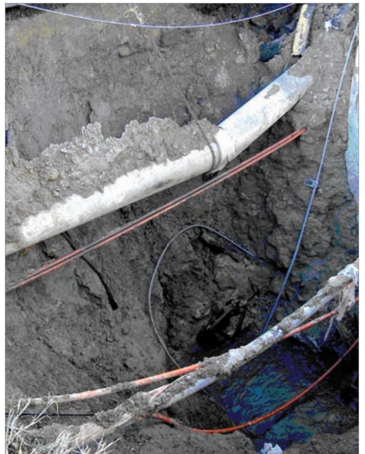
The Essen Lane collapse exposed the failure in the top of the 54-in. RCP sanitary sewer gravity main. At the top, a 15-in. potable water main is broken and numerous other utilities are adjacent, including telephone, cable and fiber optic lines.
