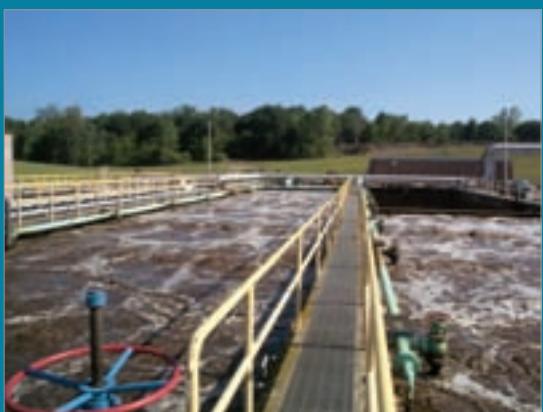
The retrofit allowed the new MBR technology to produce much cleaner effluent into the nearby Aurora Branch of the Chagrin River.
