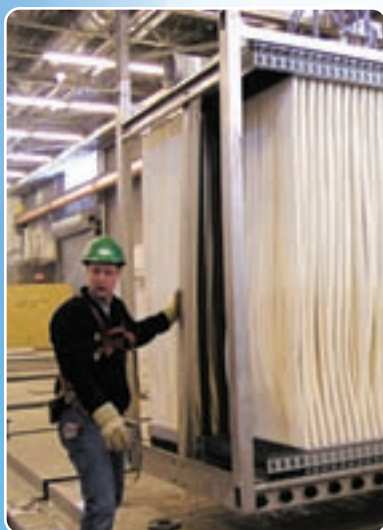
A technician installs a ZeeWeed membrane cassette into the 1.3 mgd tertiary filtration plant at Gold Bar WWTP.
