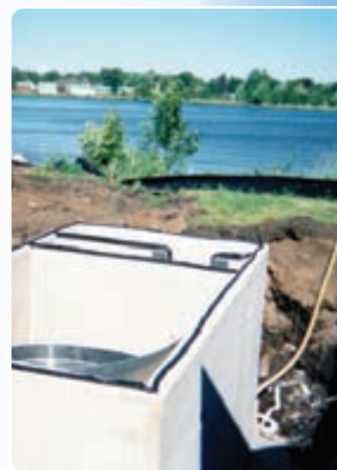
The Vortechs Model 5000 is installed in downtown Little Falls on the banks of the Mississippi River.
