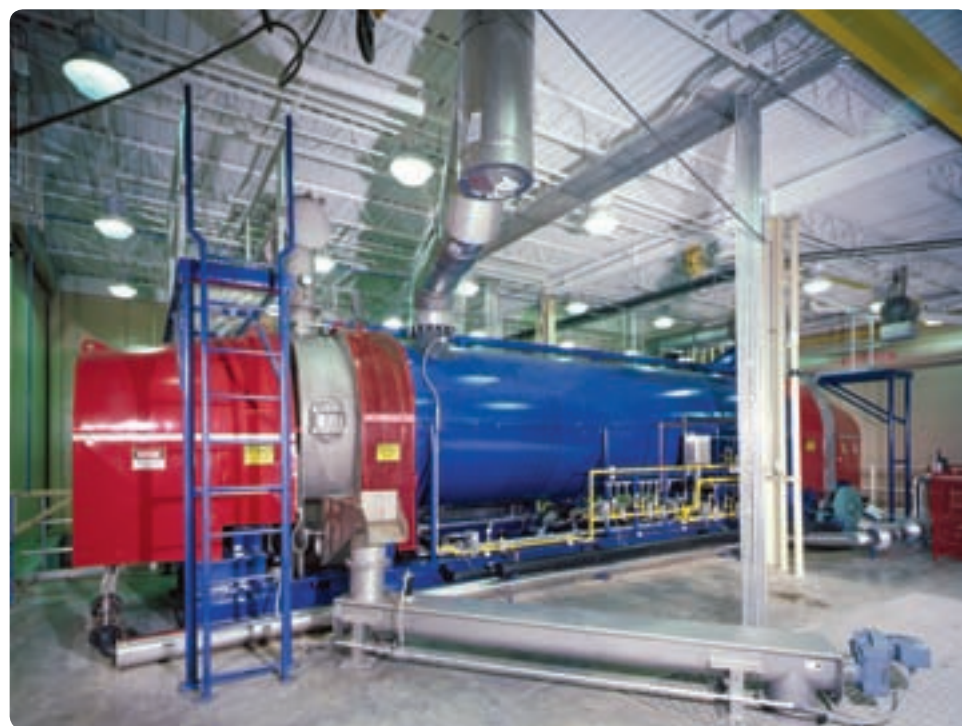
Dragon dryer system, Newport, Tenn.
