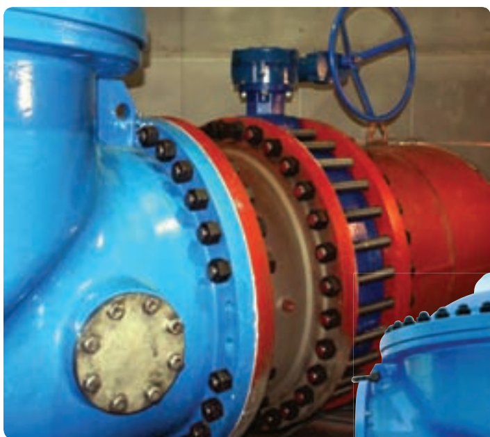
A large factory-built control valve station is made with only a single control valve
