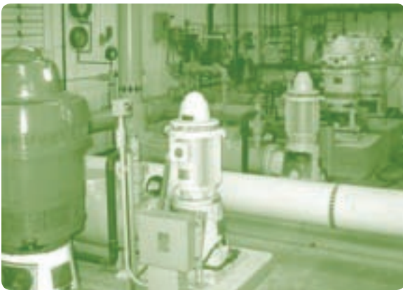
A view of the treated water high lift pumps in the town of Stockbridge Water Department's water plant.
