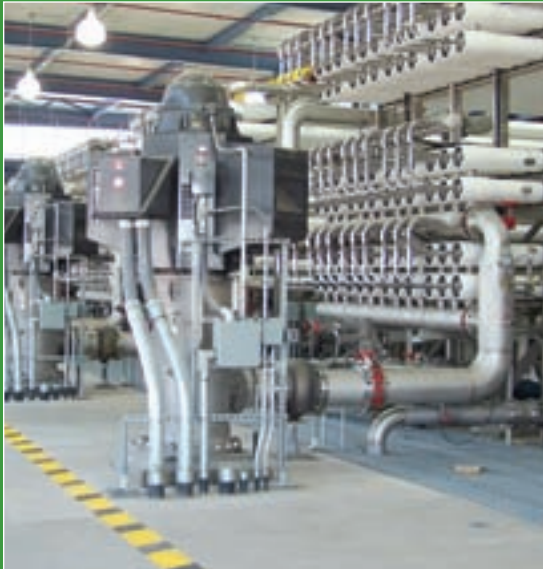
Interior photo of the membrane skids at the Kay Bailey Hutchison Desalination Plant.
