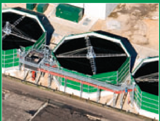
New infrastructure, including three NTFs, increased tertiary treatment capacity to keep the facility's level legal.
