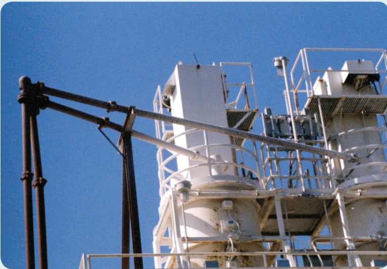
After two years of service, plant operators in Alexandria, Va., could find no hint of wear on the Smart Elbows.
