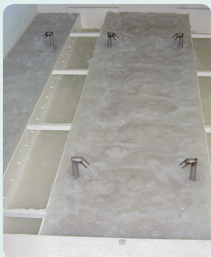
The new system started up in 2002 and has saved operator time and treatment costs.
