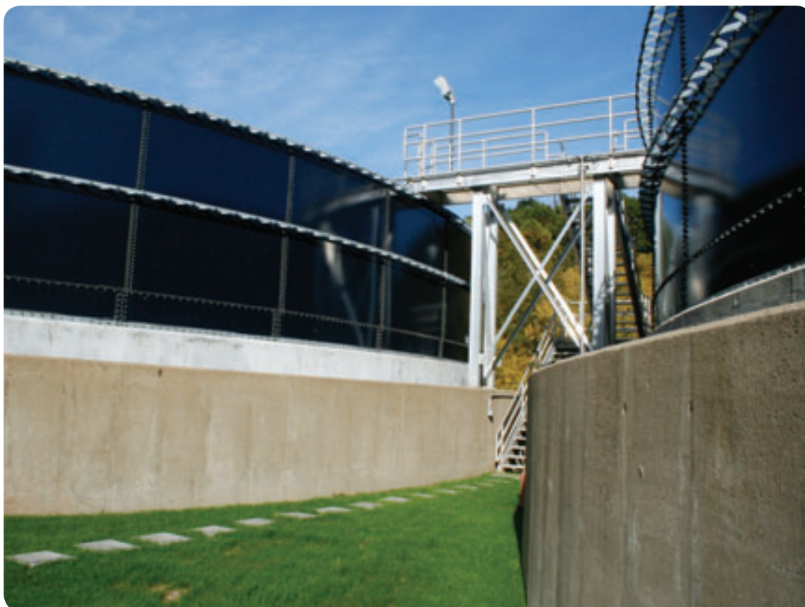
Trickling filters can help municipal agencies address SSO and CSO events.
