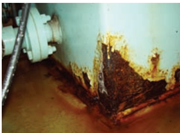
Figure 2. Rust Deterioration of a Steel Tank
