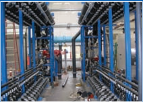
Cottage Grove funded the WTP upgrade with the help of two loans from the Oregon Economic and Community Development Department.
