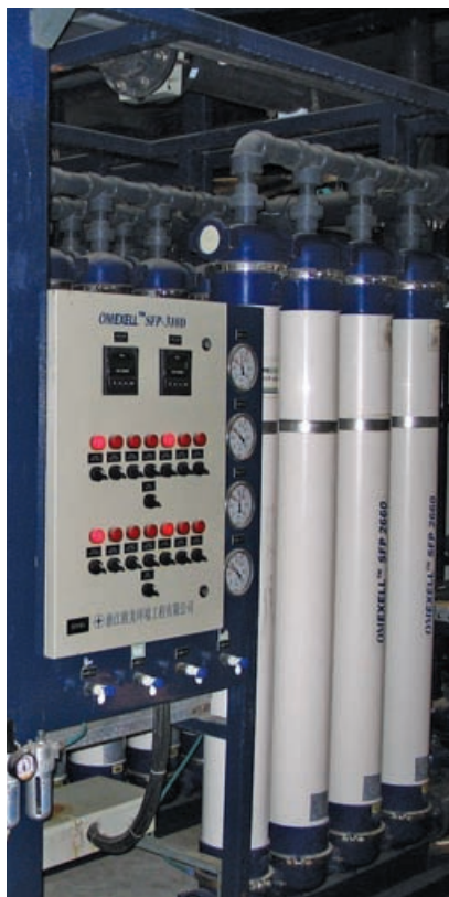
A Chinese petrochemical plant uses a combination of UF and RO to treat and reuse its wastewater. Even with this integrated solution, aggressive pretreatment and chemical cleaning is necessary due to the complex and toxic elements in the water.
