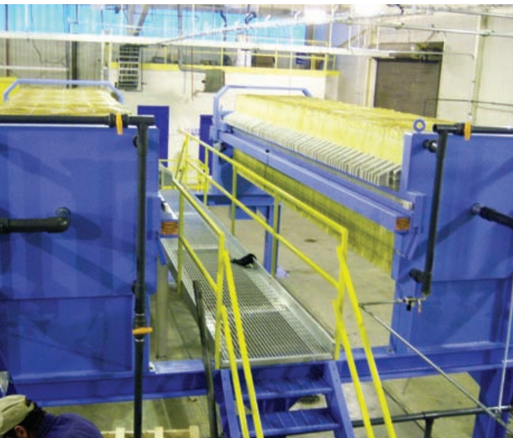
The installation included two 125-cu-ft filter presses with 1,200-mm plates.
