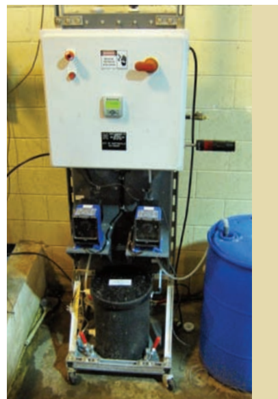
The chlorine dioxide generator is located at the head of the plant. At left is a corner of the influent trough that is dosed with the compound.
