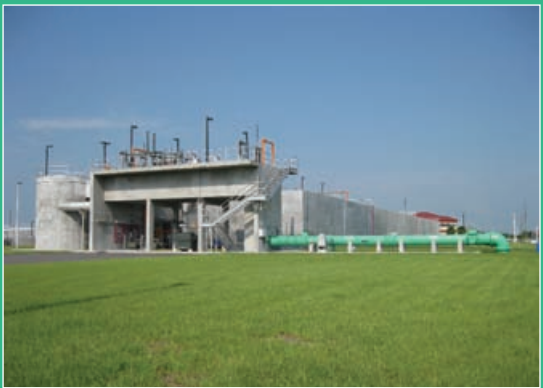
First-year performance records indicate that the 6-mgd facility may be operating at approximately 8 to 9 mgd.
