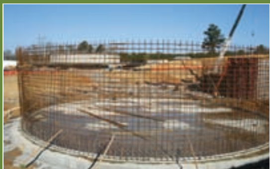
The WWTP expansion and upgrade project spanned two years and cost $14.5 million.
