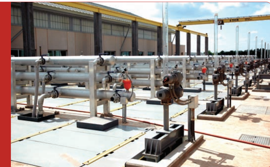
MBR technology helped BRWRF meet ENR standards and avoid adverse impacts on the region's drinking water supply. (All photos courtesy of GE Water.)
