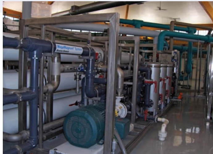
The new system's 18-in.-diameter elements process water in a smaller footprint, which allowed the city to spend $1 million less on a smaller building.
