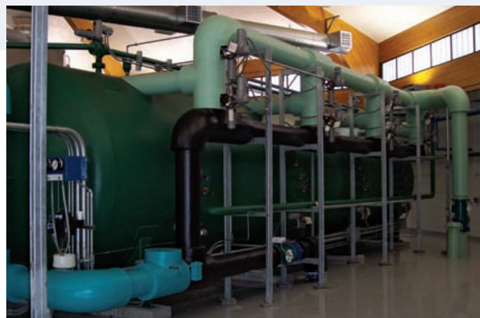
The new RO system requires minimal maintenance and the facility operator expects it will last at least three to five years.
