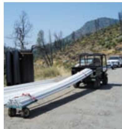
Different types of treatment and systems are being used in the area, including chamber drainfield systems. The system selection depended on location of the marina, slope and soils.
