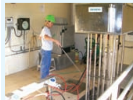
Operators can clean the new UV system in less than an hour by pulling a UV bank from the water every two weeks and hosing it off.
