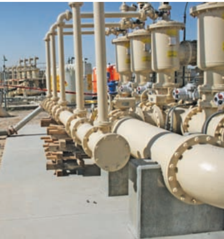
Adding automatic self-cleaning screen filters to a brackish well desalination system dramatically reduced cartridge and labor costs for the city. (Photo courtesy of Keith Edwards, city of Goodyear.)
