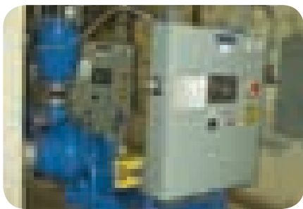
Three new 125-hp variable flow blowers replaced single-speed centrifugal blowers.
