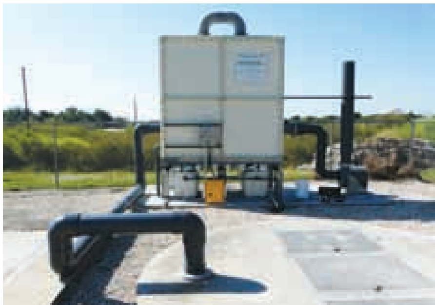
Odor complaints increased substantially at this central Florida utility, prompting officials to install a biological air treatment system. One day after installation, the system was achieving a 99% removal efficiency of H 2 S.
