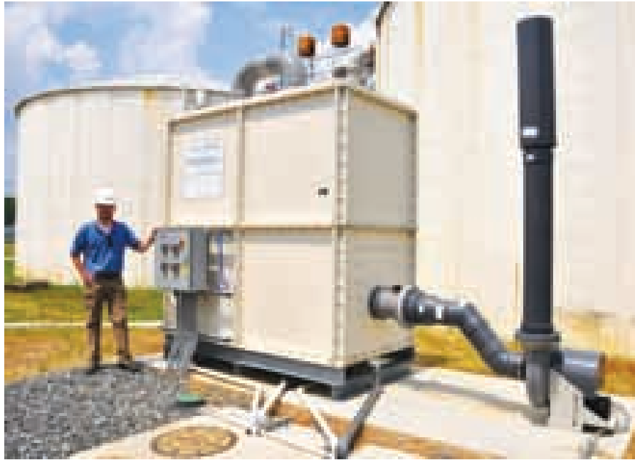
The MÓNASHELL uses naturally occurring shell media to biologically treat odorous airstreams.
