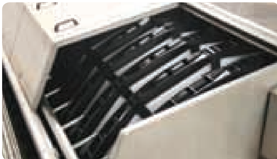
Two Kruger Hydrotech HSF2220-2F Discfilter units were installed at the Wildcat Hill WWTF.
