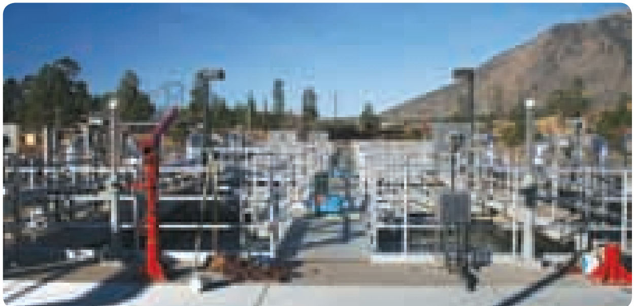
The AnoxKaldnes Hybas system consists of two trains. Each train contains an anoxic basin, followed by two oxalic Hybas basins.
