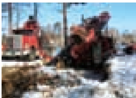
RBF technology produced a 12-mgd supply, by way of a 165-ft-long gravel well, beneath the Merrimack River in New Hampshire.
