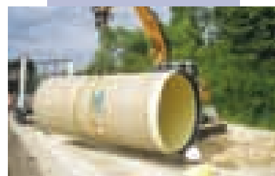
The pipe installation provided many benefits, including French Water Act compliance and the ability to conduct an open installation where the road was extended.
