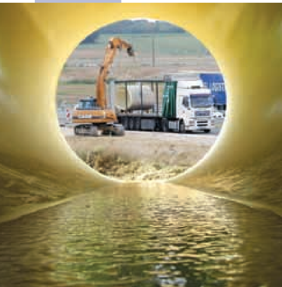
GRP pipe replaced damaged metal pipes on France's Highway A31 while additional lanes were built.
