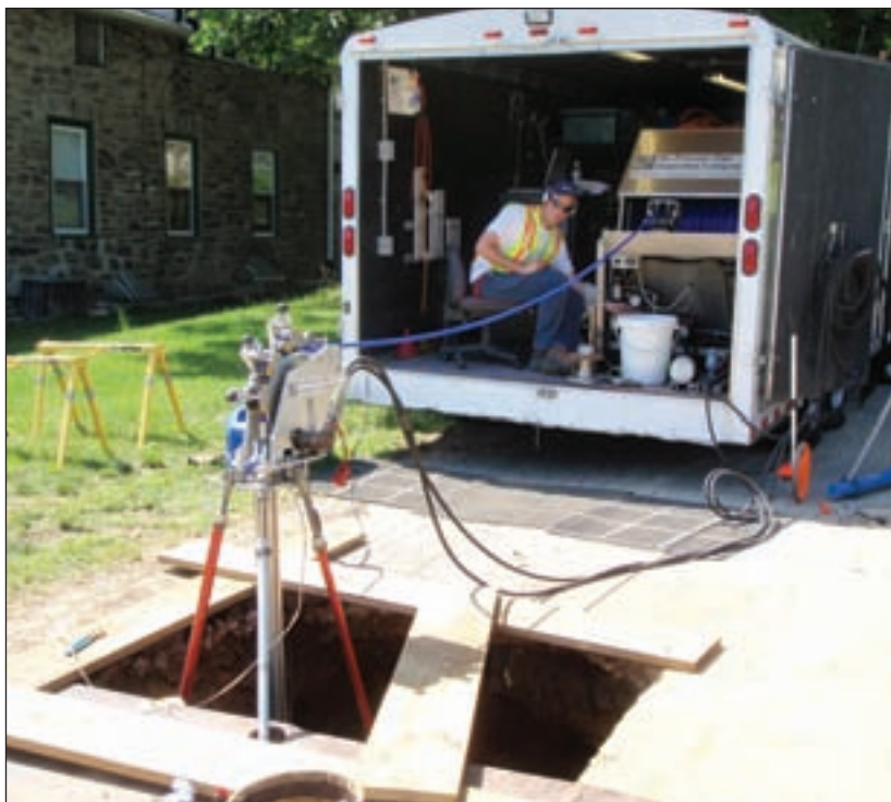
PWD staff tried unsuccessfully to locate the leak with above-ground technology before turning to Sahara, a leak detection tool designed for live inspection of large-diameter water mains.
