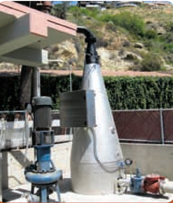
Laguna Beach installed its second ECO2 cone outside, painting the tip black so that it blends in with the surrounding landscape.
